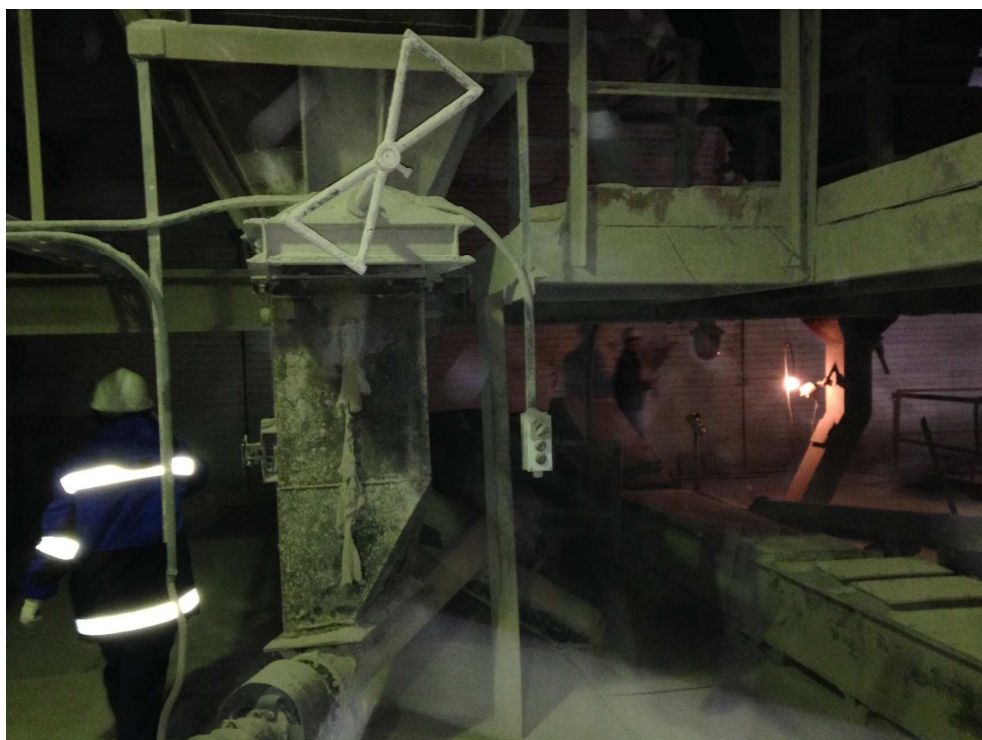
Figure 4 Dust collection from the ESP at the VCP
