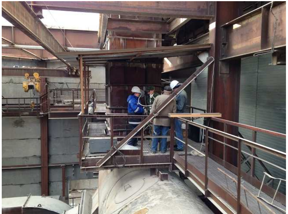
The sampling platform – the flue gas flows in downward direction
