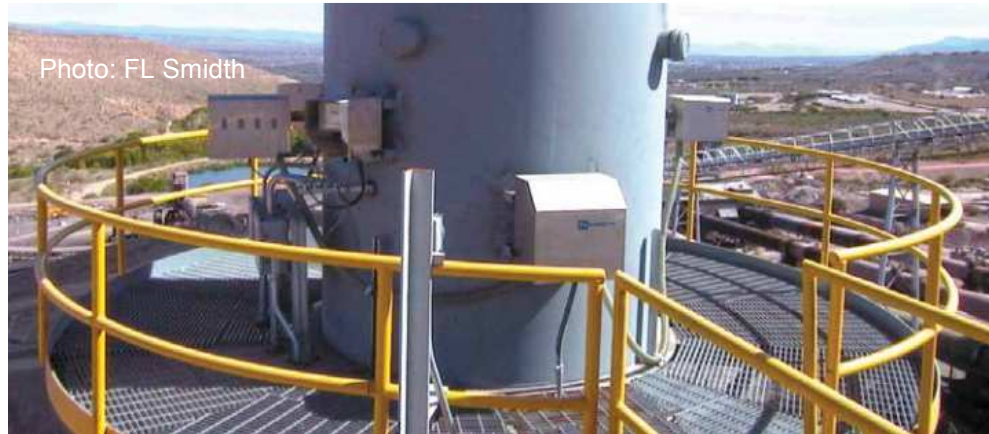
Figure 3 Example of online monitoring system for stack emission
