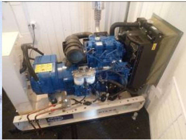
New diesel generator
