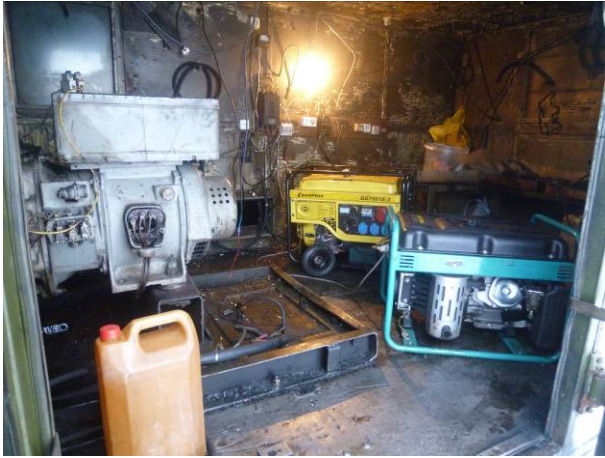
Old diesel generator
