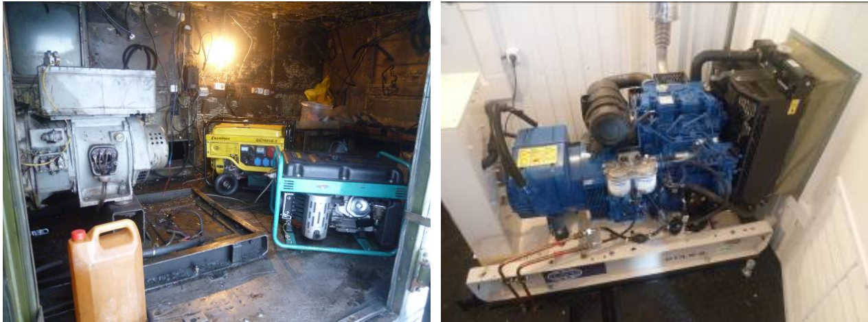
Old 10.4 kW diesel generator (left) and the new, more efficient 10.8 kW diesel generator
